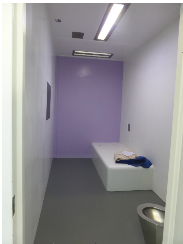
Windowless ISU cell.
