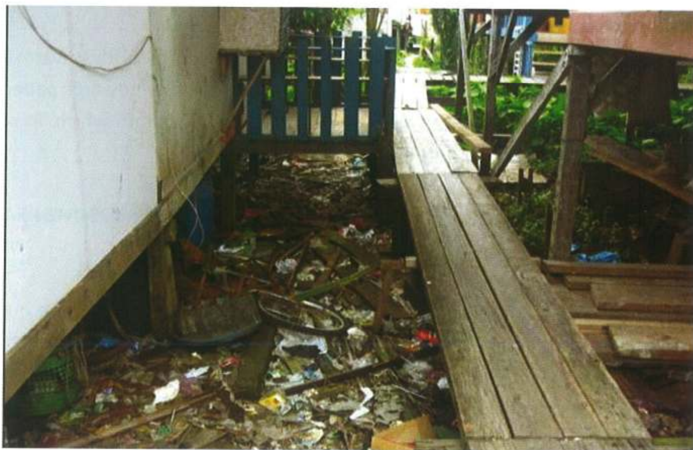
Indiscriminate waste disposal was apparent, and without access to proper sanitation and waste disposal services. The picture was taken by SUHAKAM during their visit to Kampung Beladin, Pusa, Sarawak
